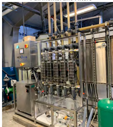
Chlorine Generation System
