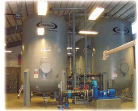
Photo: Granular activated carbon absorber filtration system
