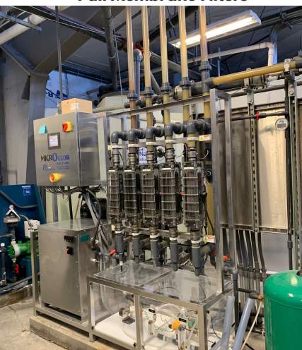
Chlorine Generation System
