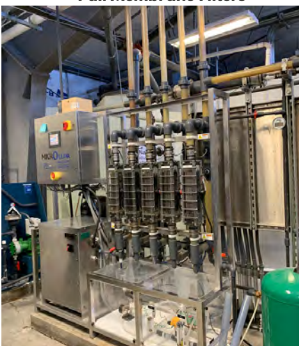
Chlorine Generation System
