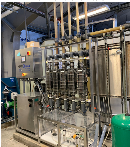
Chlorine Generation System
